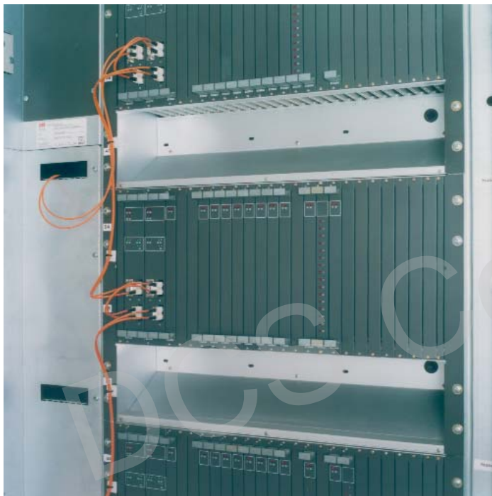
Racks within a station
